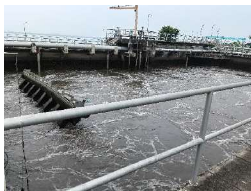
15 MLD STP at Jharkhandi Mahadev
