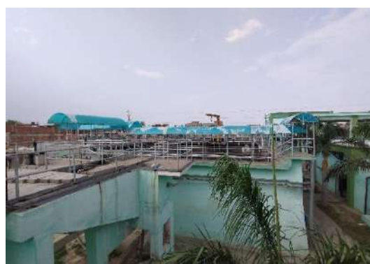
MLD STP at Jharkhandi Mahadev
