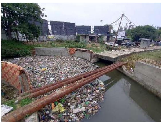
Image 4-5: Solid waste accumulated in drain at Paidleyganj Nallah, SPS
